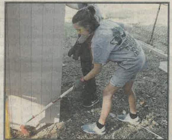
AYLA HEADRICK DIGS OUT the base of the new shed to put in a rain barrier.
