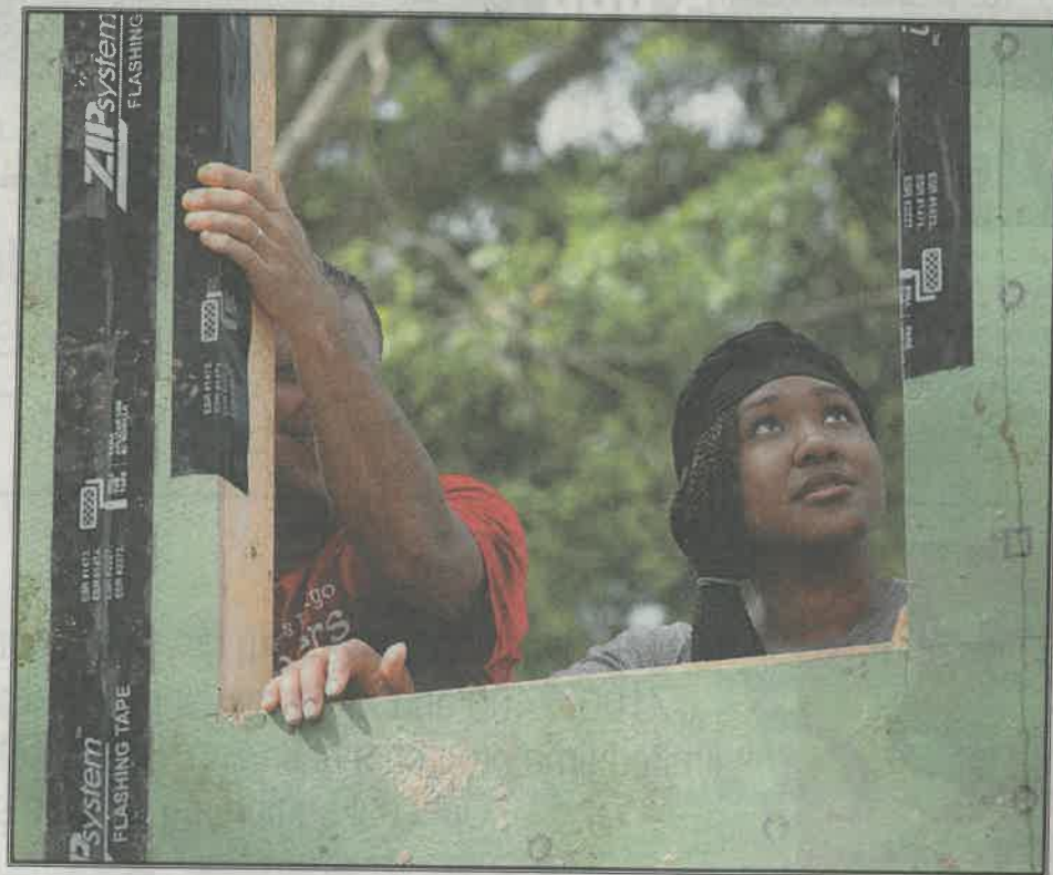
JAMEELAH MOSTELLA (RIGHT), HELPS raise the first wall of her Habitat for Humanity home on West Newcomen Street in Alcoa. She grew up just down the street.
