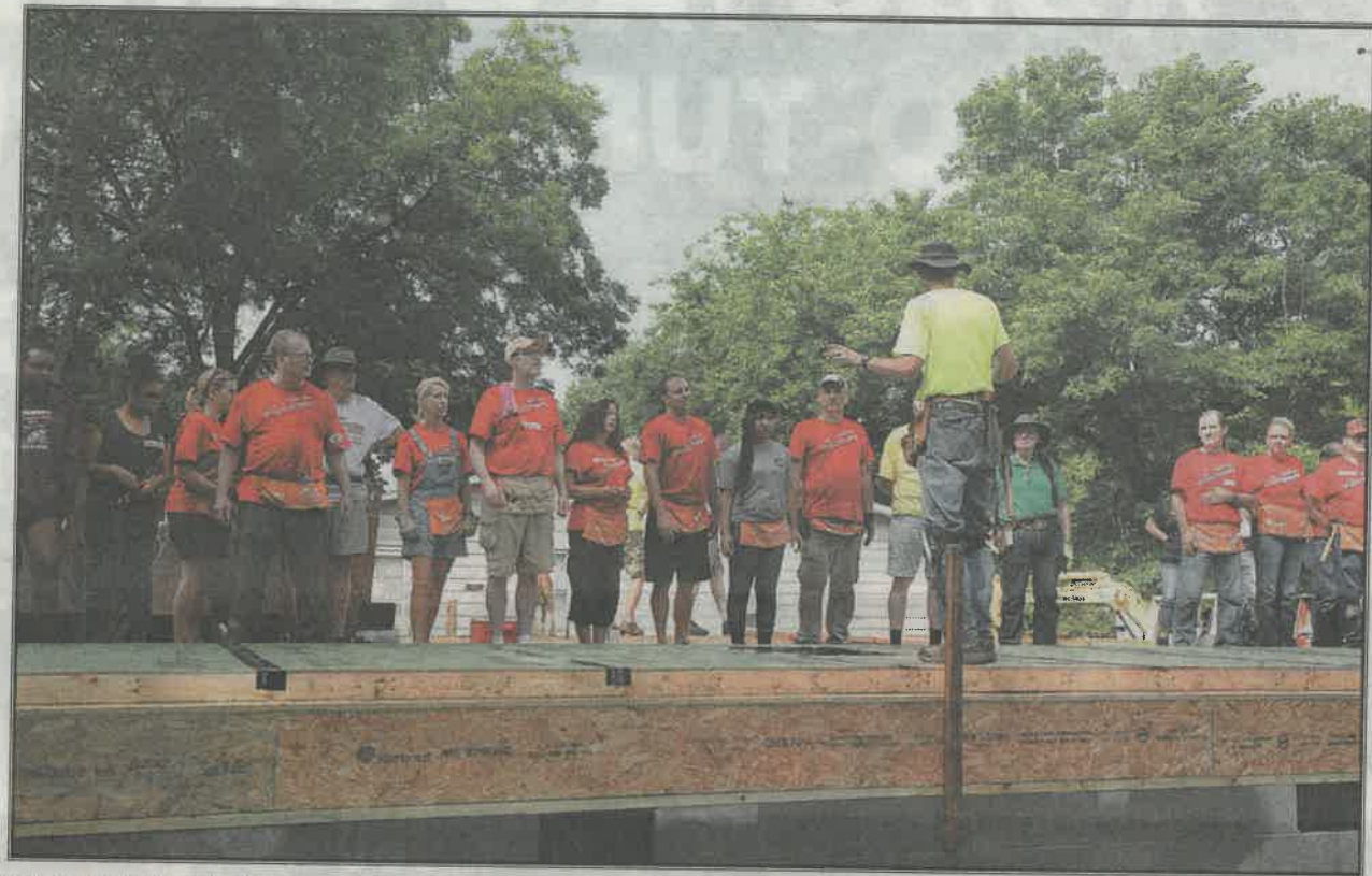
KEN SOERENSON (CENTER), GIVES volunteers instructions on how to properly raise the first wall of a Habitat House on West Newcomen Street Thursday morning in Alcoa. The house should be completed sometime in September.
