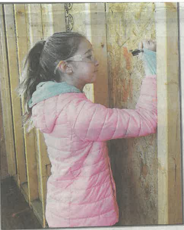
MARY RYLAN CHILDRESS WRITES an encouraging message to the new homeowner on the frame of the kitchen wall on Saturday on West Newton Street in Alcoa during a Habitat for Humanity home build.
