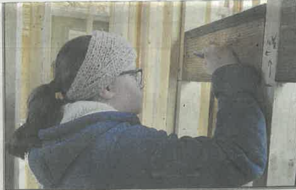
AMANDA BURKHALTER WRITES HER wishes for the new homeowner on the frame of the home on West Newton Street in Alcoa during a Habitat for Humanity home build.
