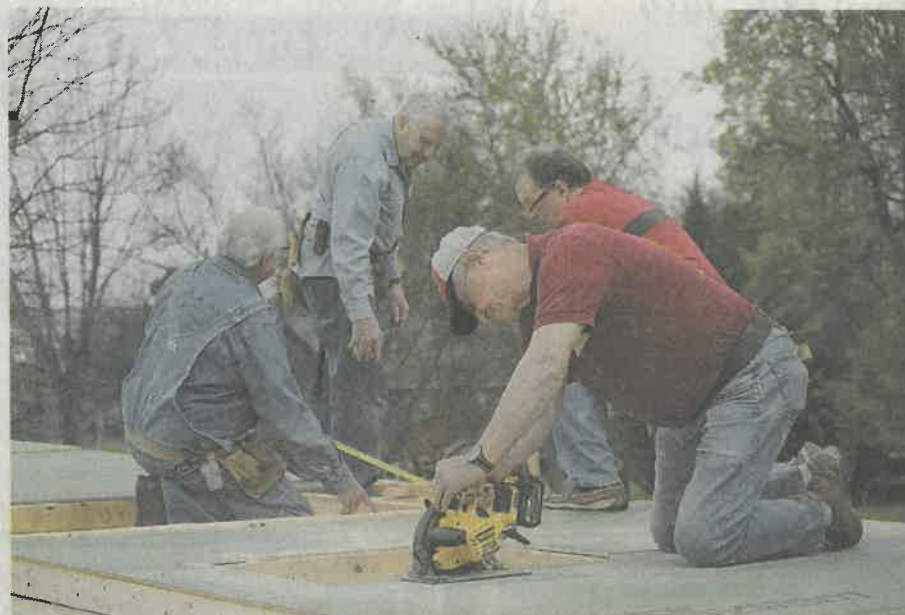
ROB STEVENSON WORKS ON constructing the walls of the home on Bessie Harvey Avenue in Alcoa. It generally takes from three to six months to complete one of the Habitat for Humanity homes. Volunteers are a large part of the process.
