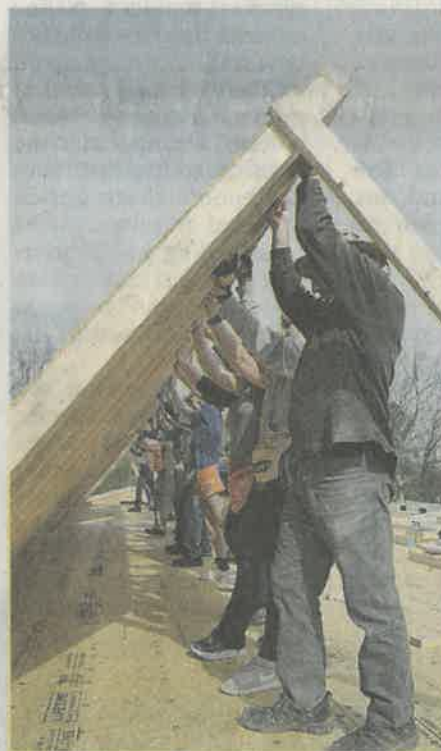
THE CREW RAISES THE first wall of the Habitat for Humanity home on Bessie Harvey Avenue in Alcoa.
