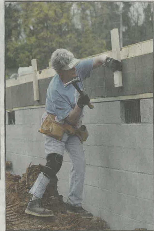
VOLUNTEER SARA GREGORY works on adding supports to raise the wall of the home on Bessie Harvey Avenue in Alcoa. She has been volunteering off and on with Habitat for more than 20 years.
