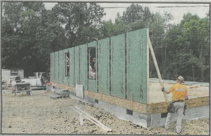
WORK IS UNDERWAY AT the Habitat for Humanity 2019 Women Build home on West Franklin Street in Alcoa.
